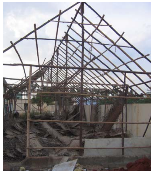
Right: Deo Gratias! The disassembling of the former shed "chapel" at the priory. For more than two years the parish Mass was held in this primitive structure. All the faithful and especially the priests were happy to see it demolished.
