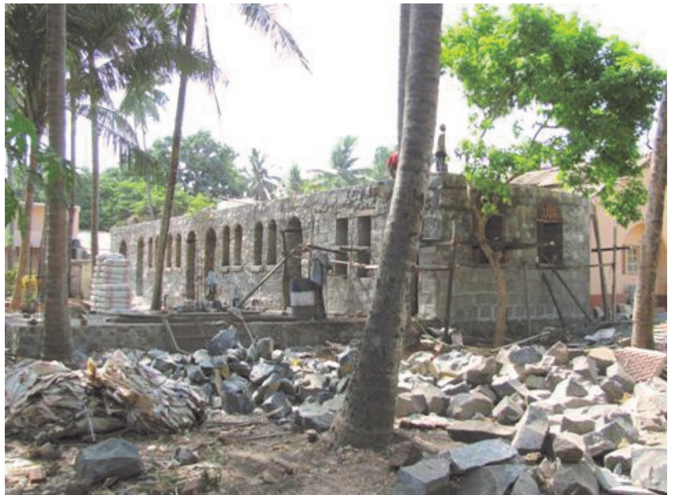
An elegant new addition to the priory takes shape at the St. Gonsalo Garcia Orphanage in the Vasai Fort.
