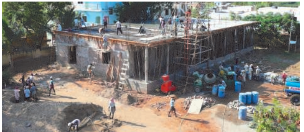
Concrete is poured on the roof of the new dormitory and study hall; the choreography of the multitude of workers was a pleasure to behold. The building will be named after the patron saint of parish priests, Saint John Vianney. All donations welcome!
